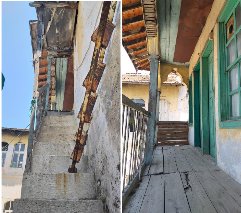
Figure 3.28. The stone stairs leading to the first floor of the Mass B, and the corridor in front of the rooms (Author, 2022).
